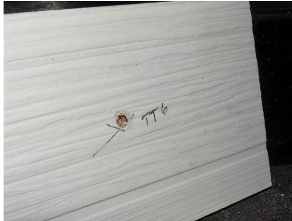
Figure 4. Typical Screw Pull Through Failure for thick siding.
