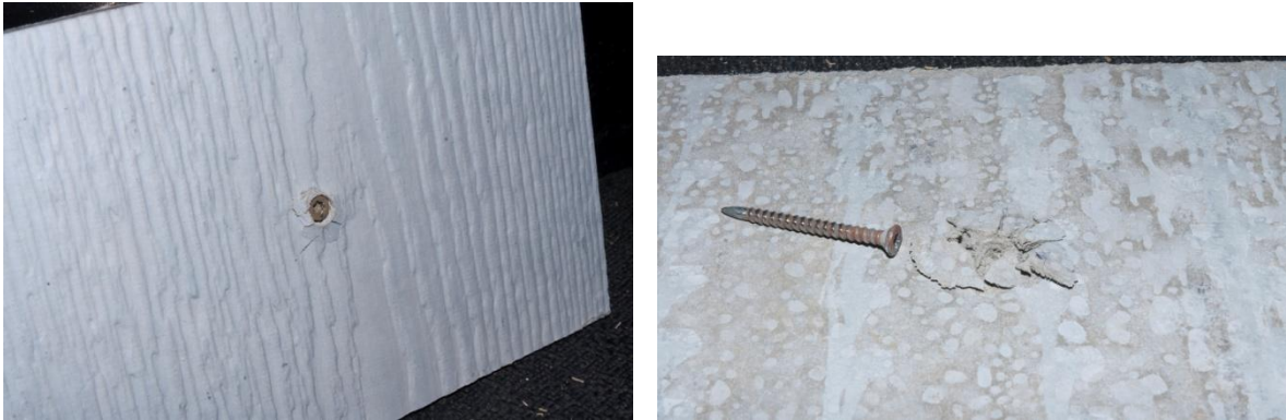
Figure 3. Typical Screw Pull Through Failure for thin siding.
